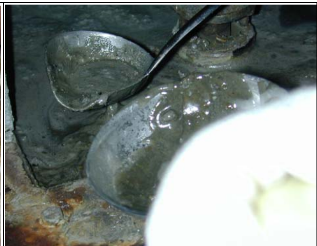
2.1.2 A scoop is cleaning sludge/foam
